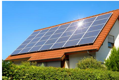
Figure 1. 7 Photovoltaic panels (electricity generation )
