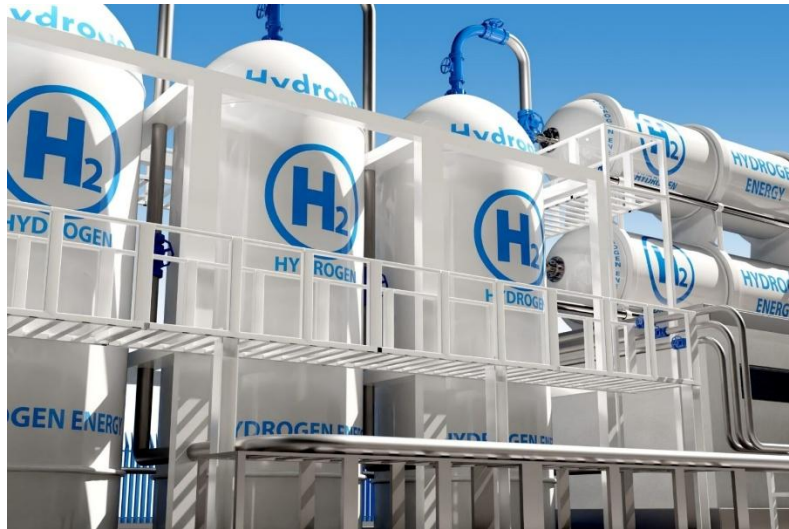
Figure 3-2 : Hydrogen gas storage source ( https://www.gexcon.com/resources/blog/hydrogen-fireball-in-a-storage-area-using-effects/ ) accessed on 17/12/2025
