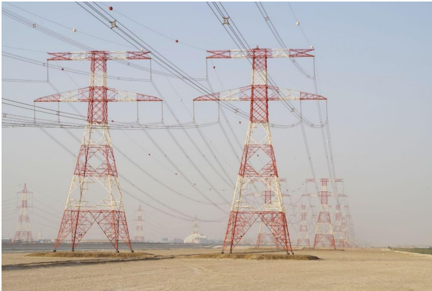
Figure 2. 5 High voltage equipment to supply electricity.
