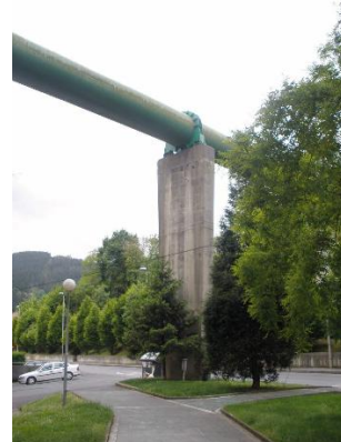
Locally above-ground gas pipelines
